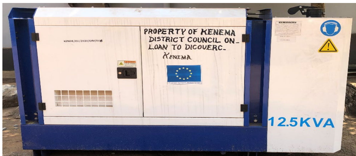
(Photo showing generator procured by the Council and installed at the Quarantined Centre)
